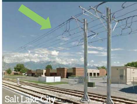
Overhead Catenary System - Wires
