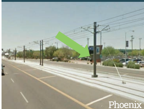
Overhead Catenary System - Poles
